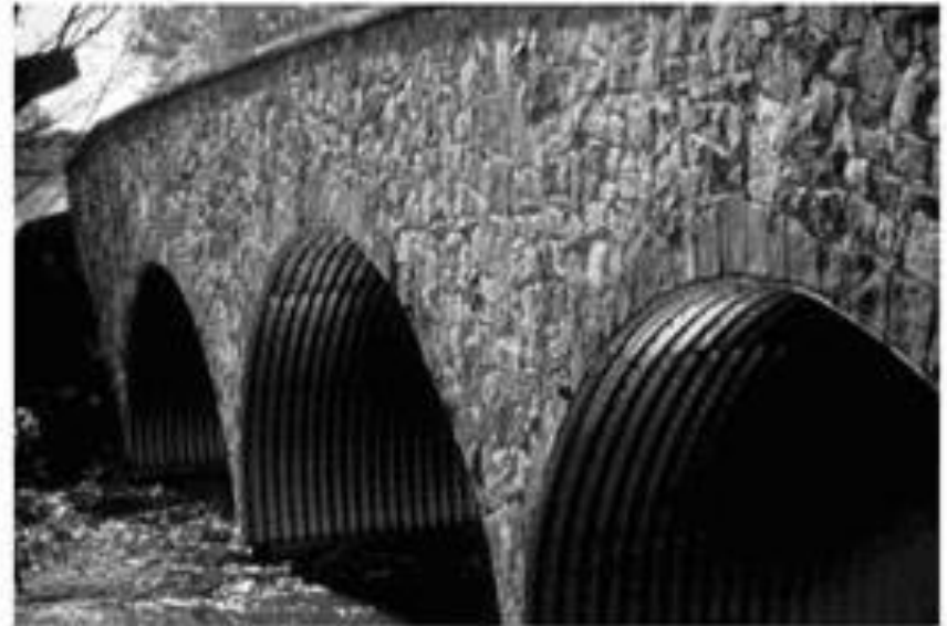
Arch Metallic culverts
